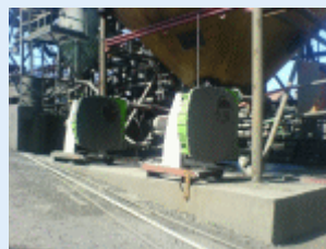
The VF65s installed at Transvaal Gold Mining Estates handle slurry at an SG of with a flow rate of m 3 /hour at 35 RPM
